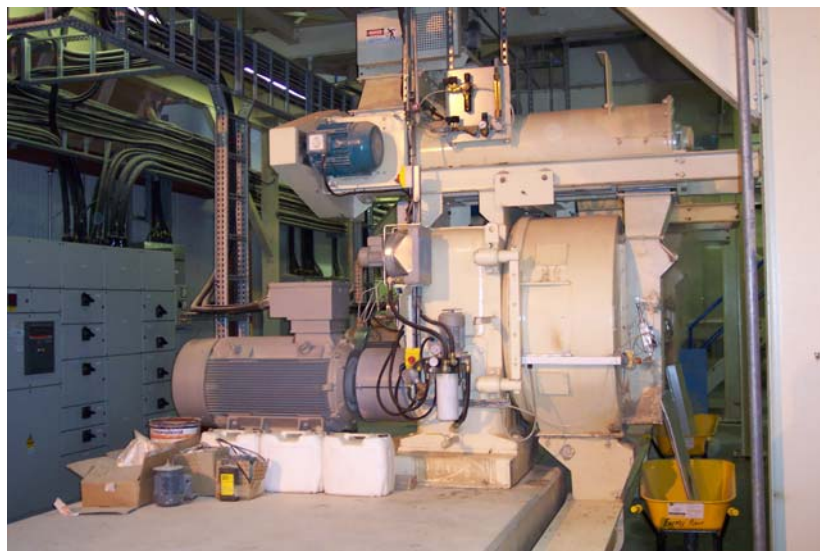
Figure 4-13: Pellet Mill at Balcas Pellet Factory, Northern Ireland
