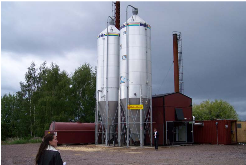
Figure 4-4: Wood Pellet Fuelled Central Heating Plant in Sweden
